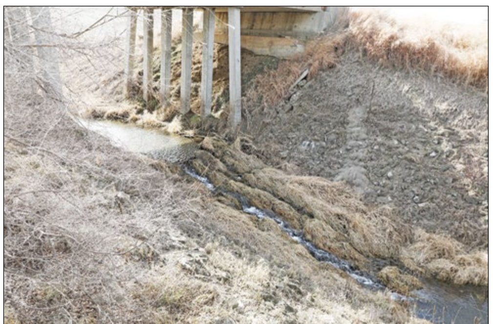
Erosion control on the waterway under the bridge will be part of the replacement project.
