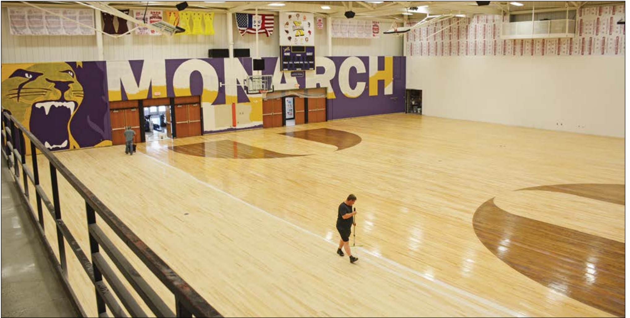
Workers from Beebe’s Hardwood Floors, of Waukee, put a coating on the gym floor at Denison High School on Tuesday. Some of the new bleachers were scheduled to arrive on Wednesday. While the bleachers are being put into place, the floor contractor will temporarily stop work, and painting of the walls will be completed. Substantial completion of the gym is expected in early September.
