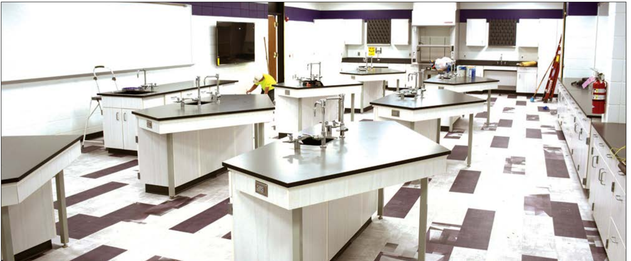
Badding Construction is wrapping up work on the three science labs – physics, chemistry and biology. The lab renovations offer more hands-on experience for students.
