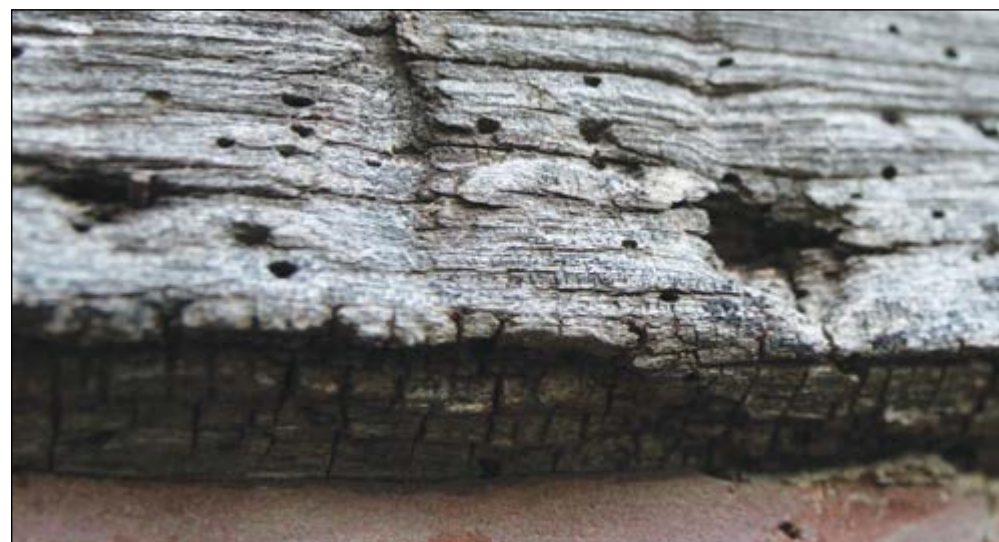
The wood of the Bell Cabin is showing signs of rot and insect damage. The wood will have to be treated to preserve it for the future.
