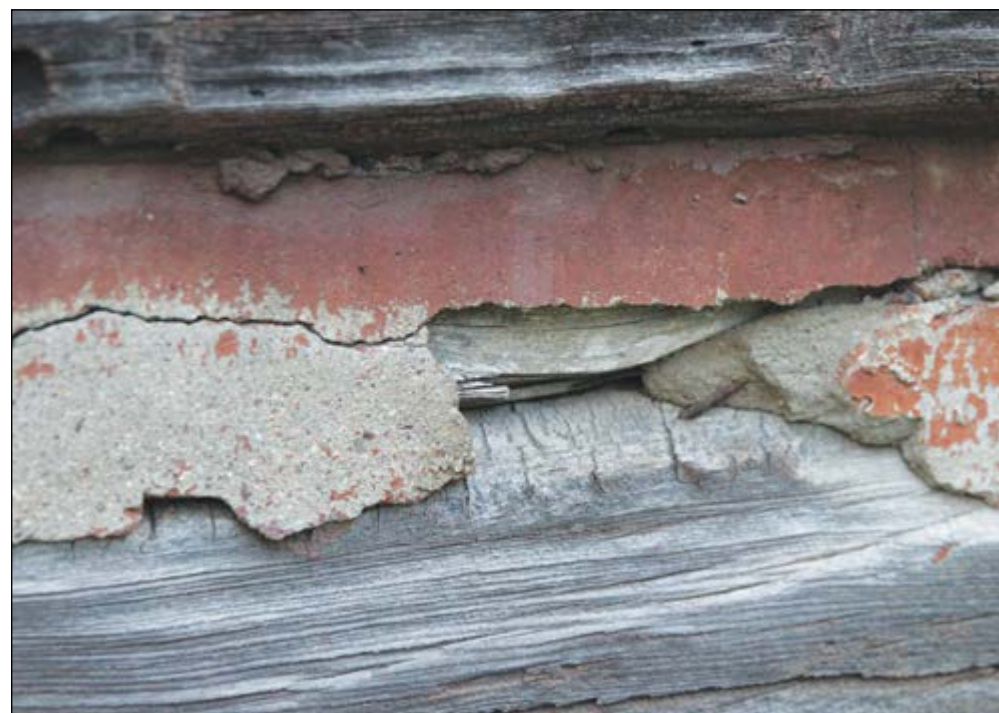
The mortar applied to the cabin at some point in the past is of a modern cement type that is crumbling – and also damages the wood during the freeze/thaw process.
