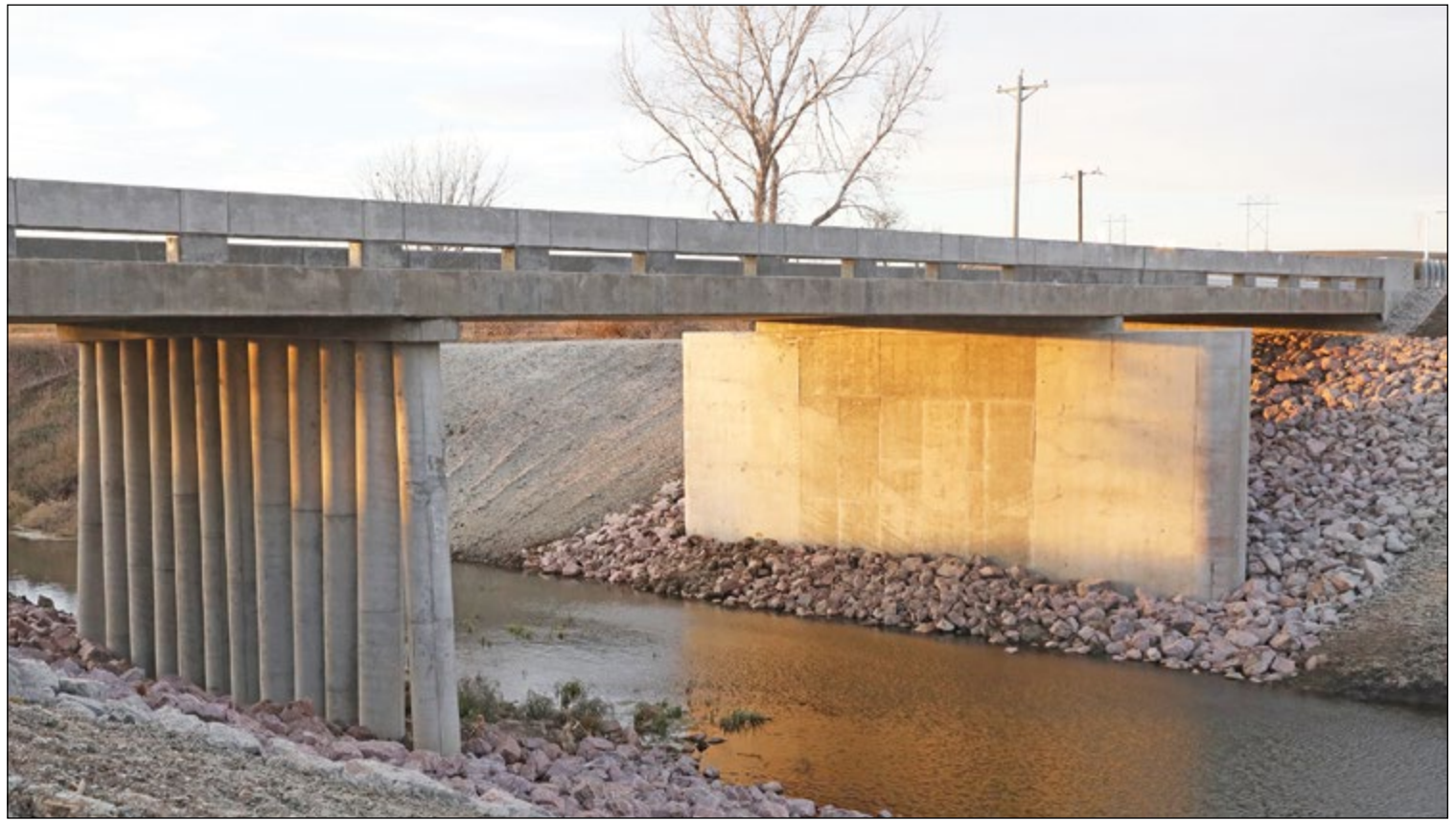
A solid beam of concrete encases all of the bridge's north pilings, which had been placed incorrectly to carry the load of the bridge.
