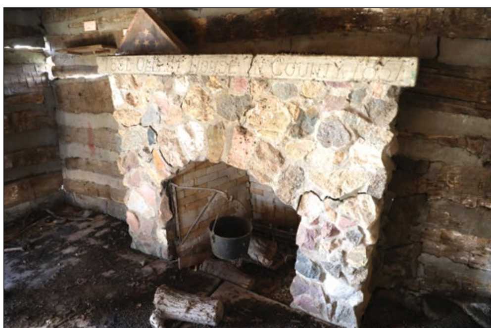
The cabin's fireplace can't be saved in its entirety; some of the fieldstone could be removed and reused, or a new fireplace could be constructed.
